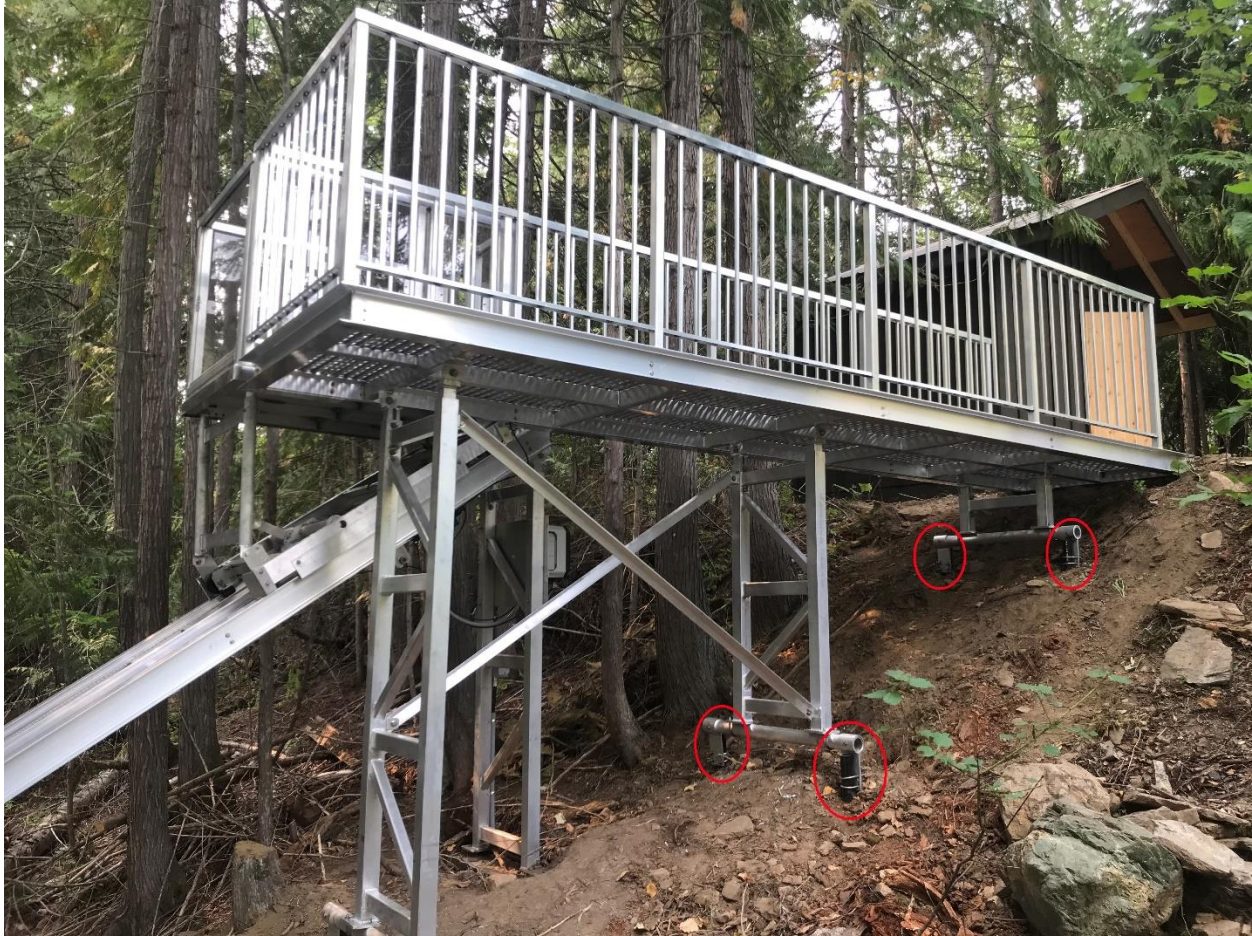
Photo 11. View of a tower bracket on two piles and their minimal permanent footprint.
