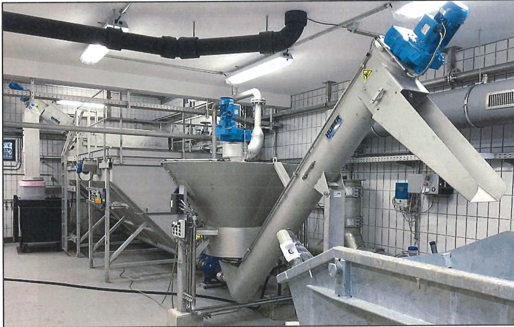
Figure 16: A typical grit removal system
