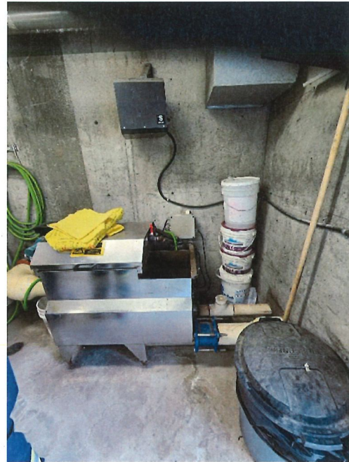
Figure 11: Vintage Views WWTP: Mechanical effluent screen inside the control room
