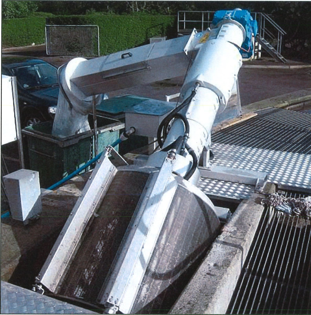
Figure 15: Typical rotary drum screen installation
