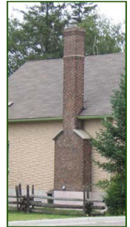
Outside chimneys do not function well.
