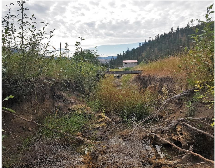
Photo 10.2 Bank erosion on Park Rill Creek in Sportsmens Bowl Road area. Photo source: NHC, Aug 2020
