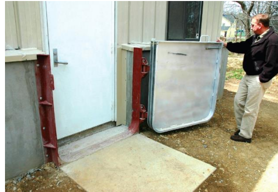
Figure 10.3 Example of a dry floodproofing barrier at a machine company
